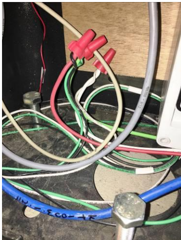
Photo 7-Supply Wiring Before Seal-Tite Protection
