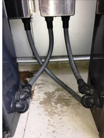
Photo 10- Supply Raceways to Vending Machines
