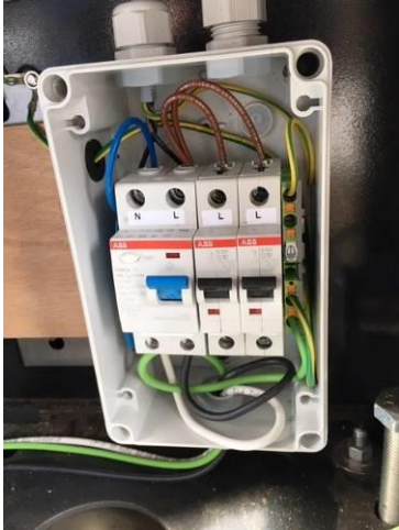
Photo 9- Internal Breaker Box
