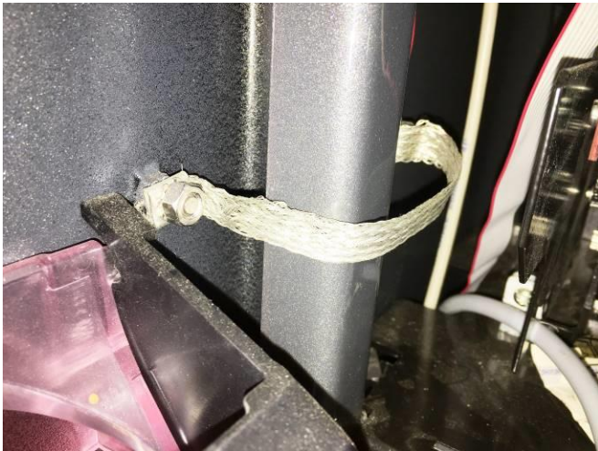
Photo 11- Door Bonding Strap
